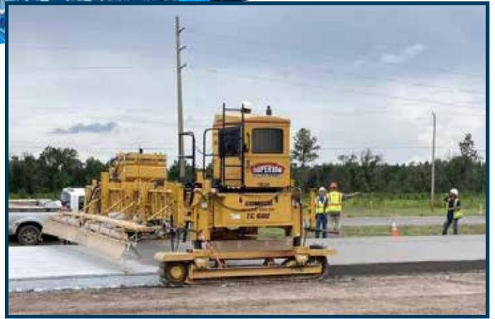
The U.S. 301 Concrete Test Road is FDOT’s only full-scale concrete testing facility in the Southeastern United States. It serves as a field laboratory for testing concrete pavement and base designs under live traffic loads. Photo courtesy of Superior Construction.
