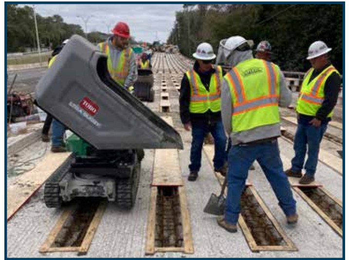
The Arlington (Fla.) Expressway Project team utilized ultra-high-performance concrete to interconnect existing precast bridge slab panels, obtaining 15,500 psi within 24 hours. Photo courtesy of Superior Construction.
