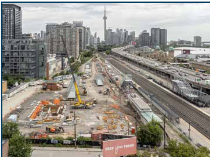
The 10-mile Ontario Line subway project through downtown Toronto. Photo courtesy of HDR.
