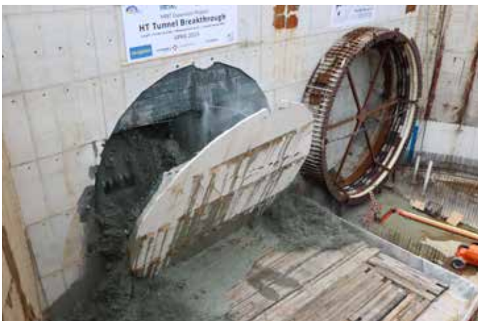
The tunnel boring machine nicknamed Mary broke through the headwall April 17 into a receiving pit on North Island, achieving a major milestone in the Hampton Roads Bridge-Tunnel expansion project.
