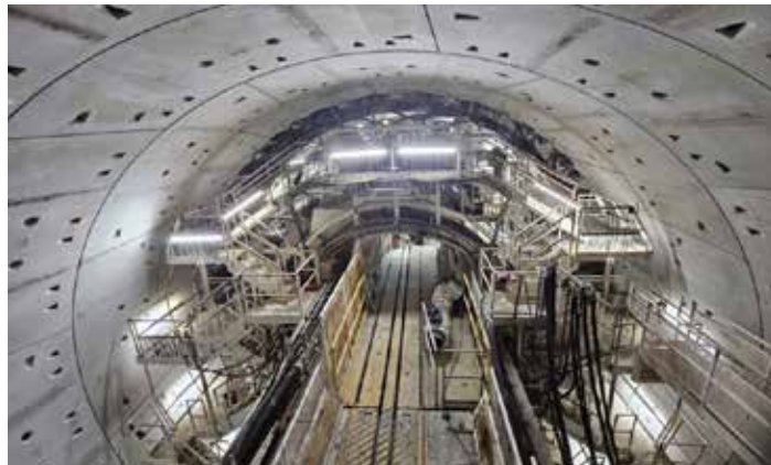
The gantry of Mary inside the tunnel where she placed the new concrete rings.
